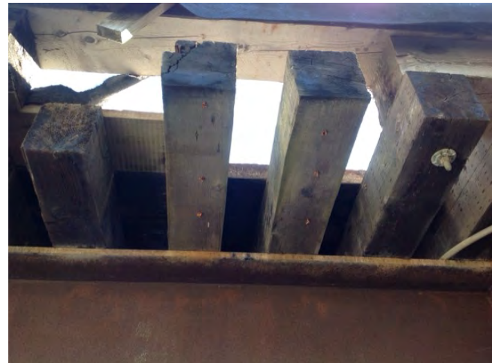
2 non-creosoted ties on right approach - replace
