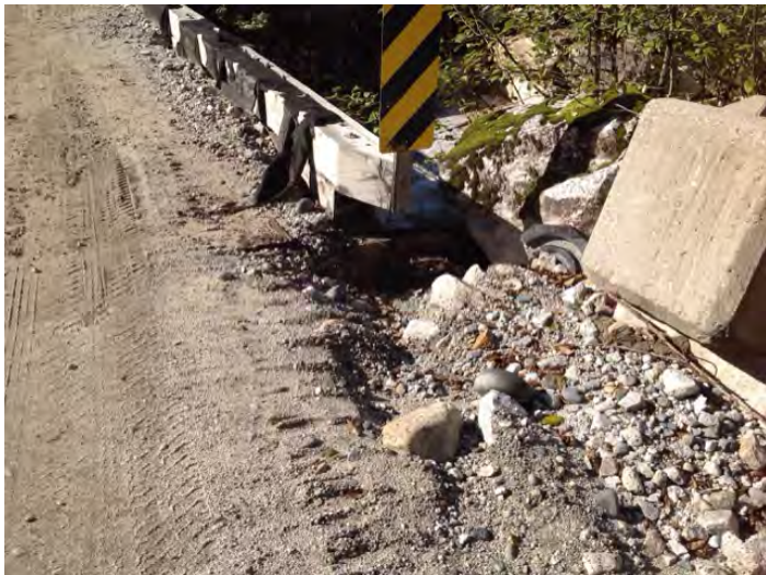
eroding fill on left upstream approach
